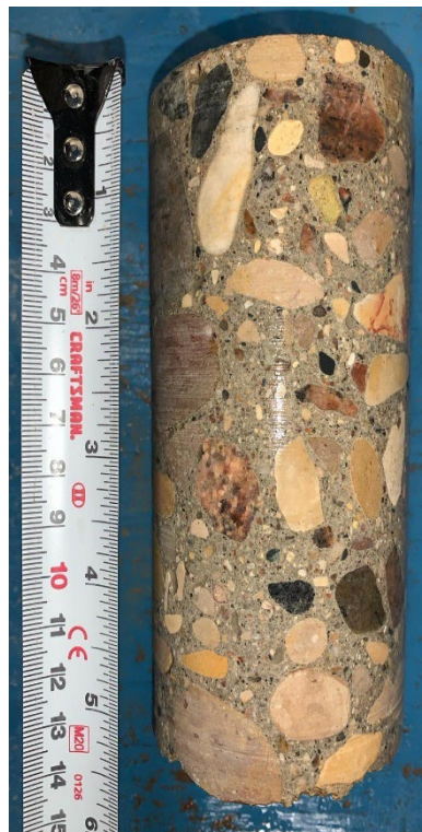
Figure 19 – Core No. 58 (Fortier Ave)
